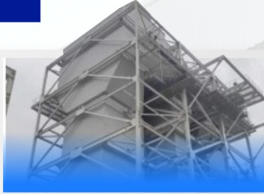
Flow Gas Duct
